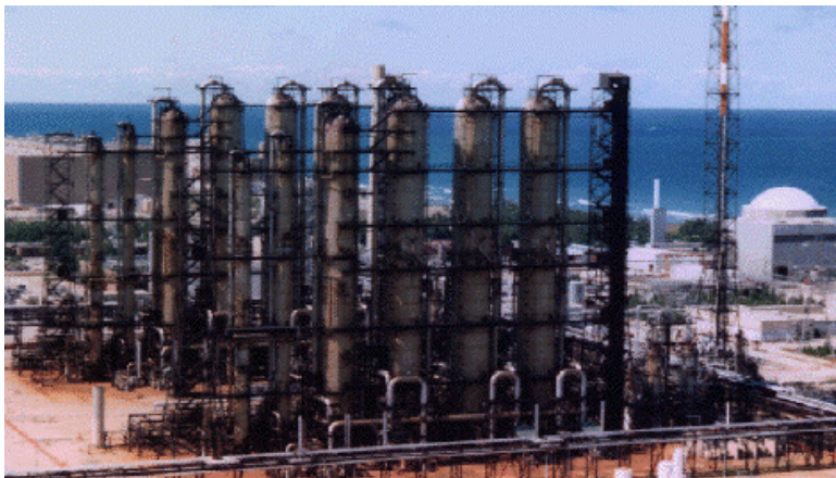
Figure 2.5. The Ontario Hydro International Bruce Point Heavy Water Plant had the capacity to produce 800 tons of per year. It was shut down in 1997. Eight plants of this size could supply enough heavy water to generate all of the energy now consumed in the world.
